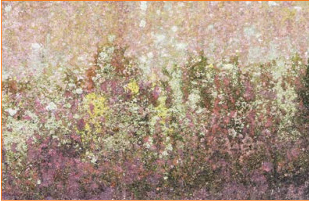
Figure 23.14 Lichens covering stucco on rear wall of South Square Market, which fronts on South Street. Air pollution suppresses the diversity of lichens, but some lichens thrive in it.
